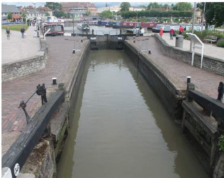
A typical river or canal lock at Stratford upon Avon. In this case the gates are operated by hand. The ones nearest the observer are open, the others are closed.
