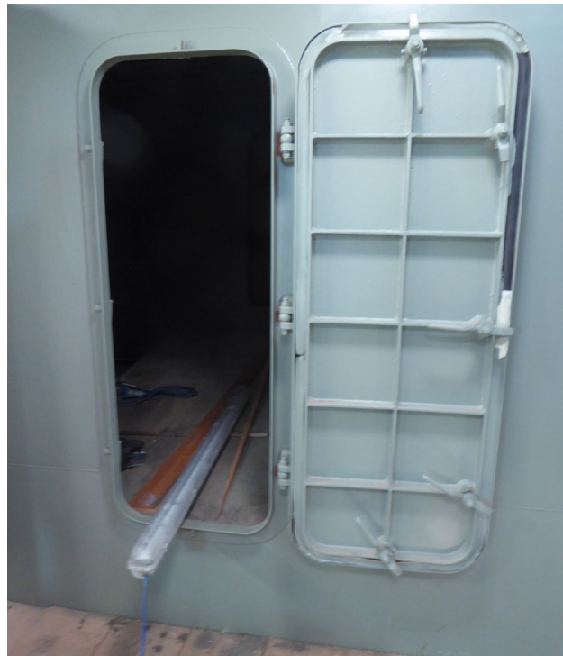
Typical raised door thresholds
